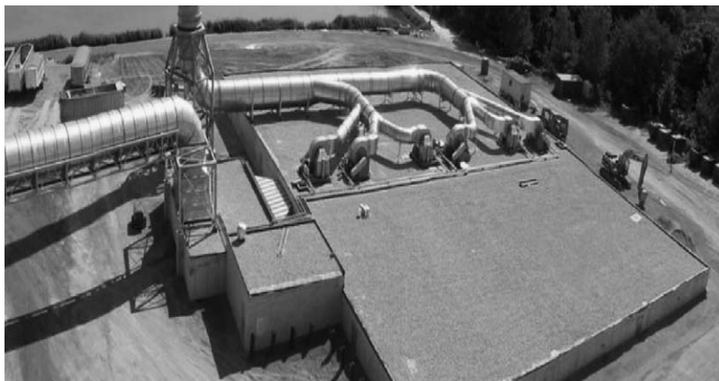
Fig. 2. A 250,000 cfm biofilter system at a rendering facility, Ontario (courtesy of Biorem Technologies Inc., Ont., Canada).
